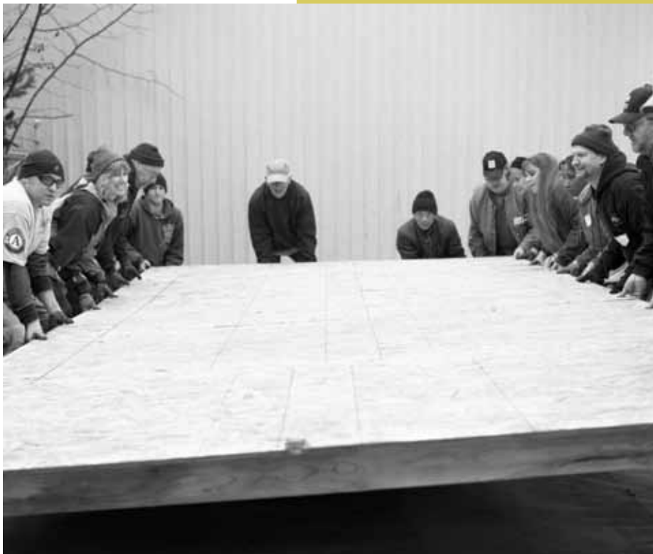
Homeowners from the southeast Martins Street community help raise the walls of their homes with volunteers on a cold January day.
